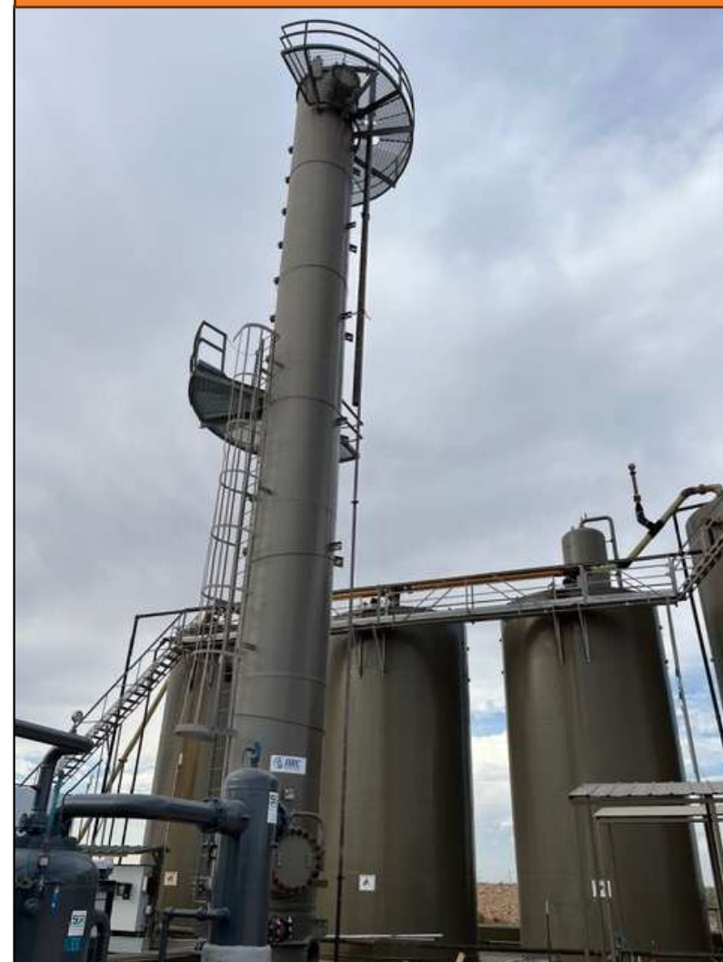
Oil H 2 S Treatment – Contact Tower
