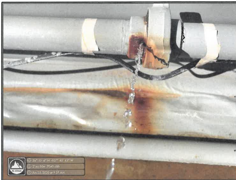
Photo 1: View of Leaking Line
