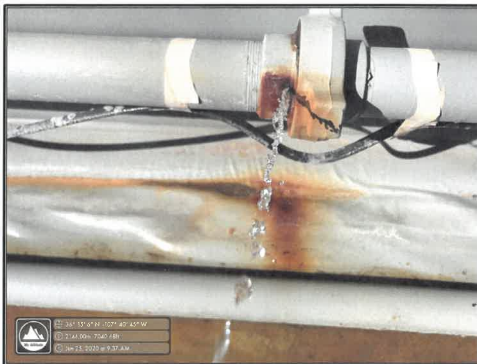
Photo 1: View of Leaking Line
