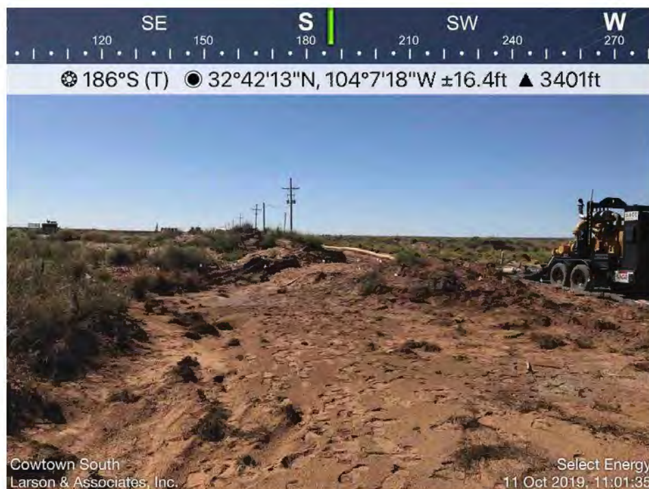
Spill area viewing south
