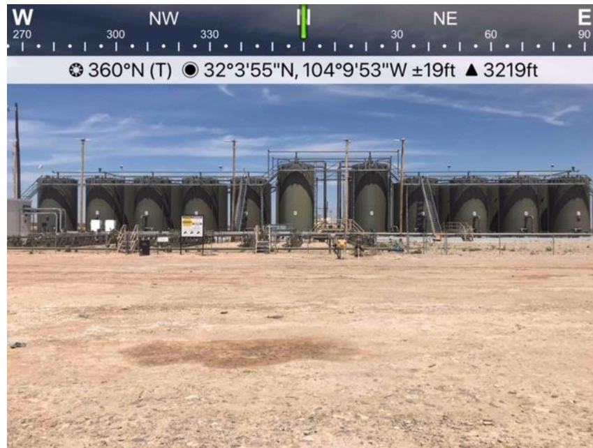
Spill area viewing north
