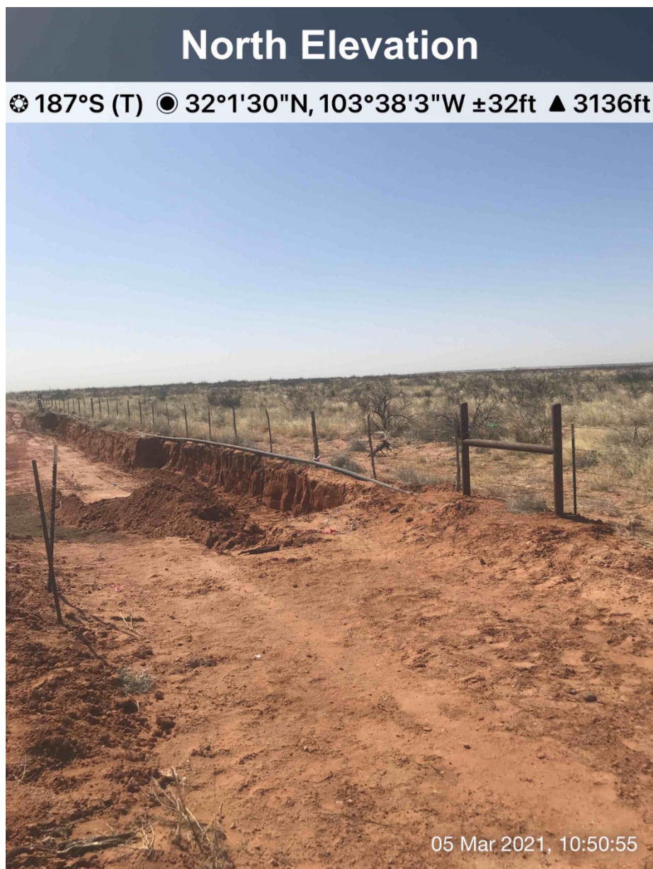
Excavated soil along the fence line at sample location C-27 and C-29, March 5, 2021
