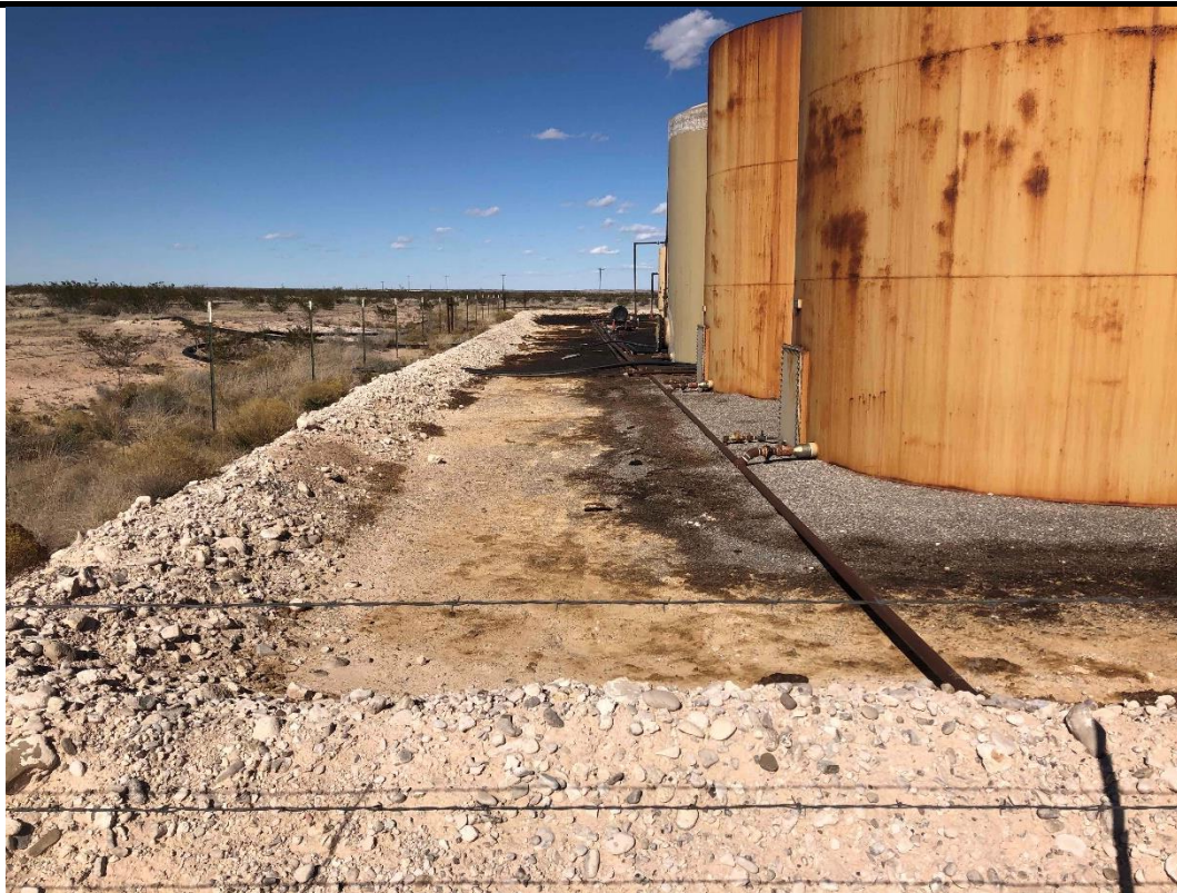
PHOTO 2: View of impacted area west of tank battery, facing north. 10/24/2019
