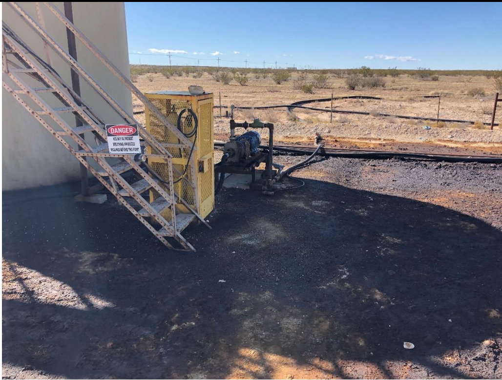
PHOTO 7: View of impacted area around VRU, facing west. 10/24/2019
