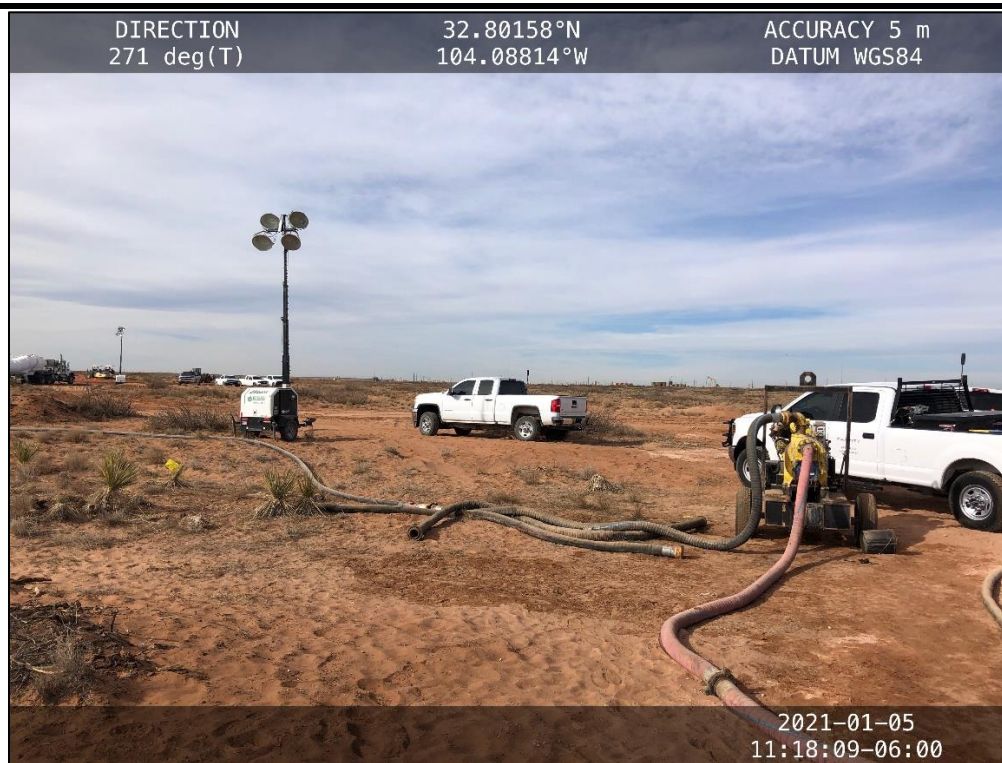
PHOTO 4: View of disposal setup at seep.
