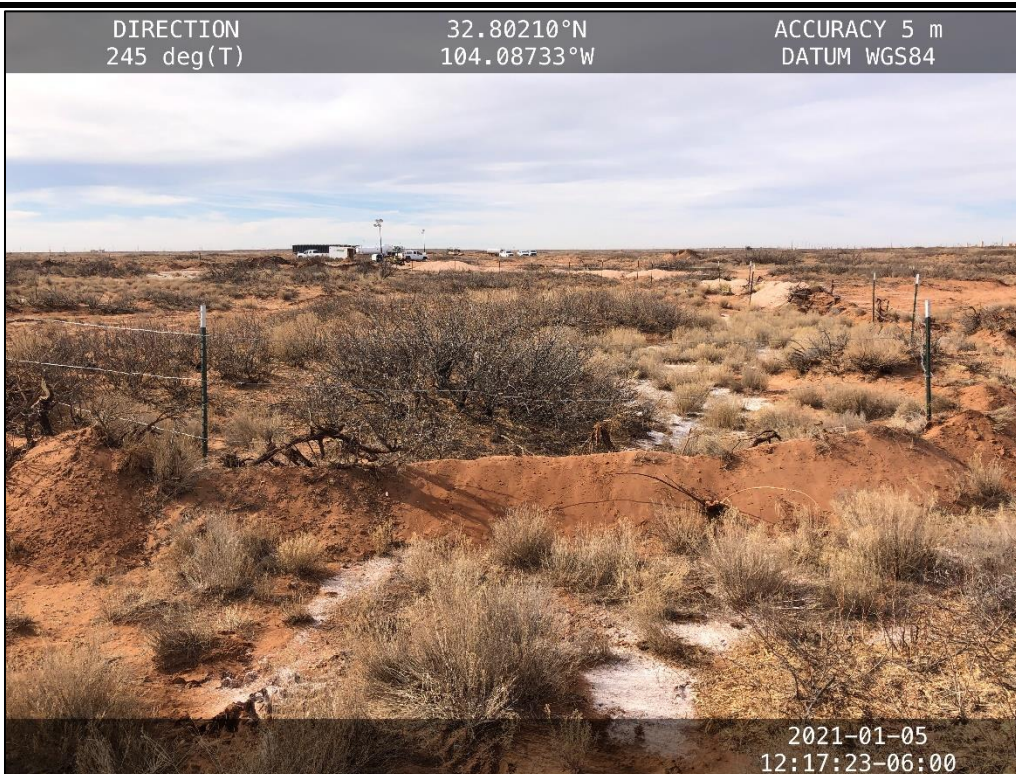
PHOTO 12: View of seep impacts
