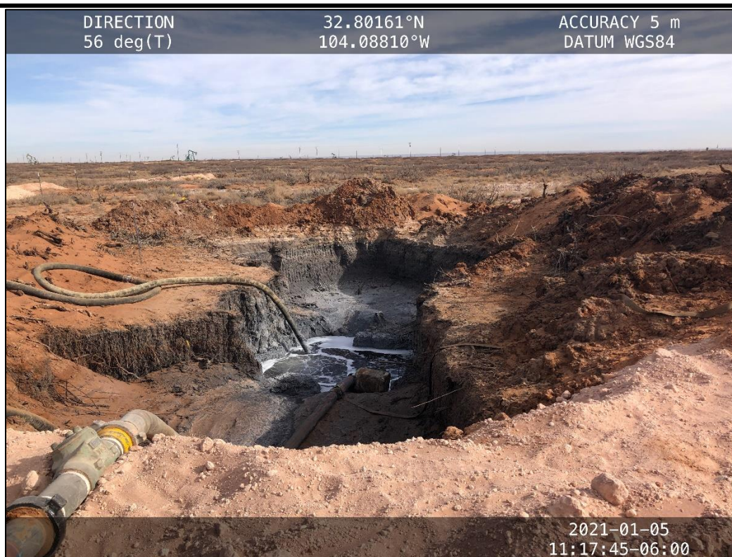
PHOTO 1: View of seep and sump
