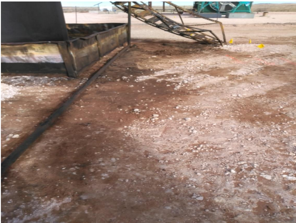
Photo 6: View of soil staining along the day tank's eastern containment wall facing north
