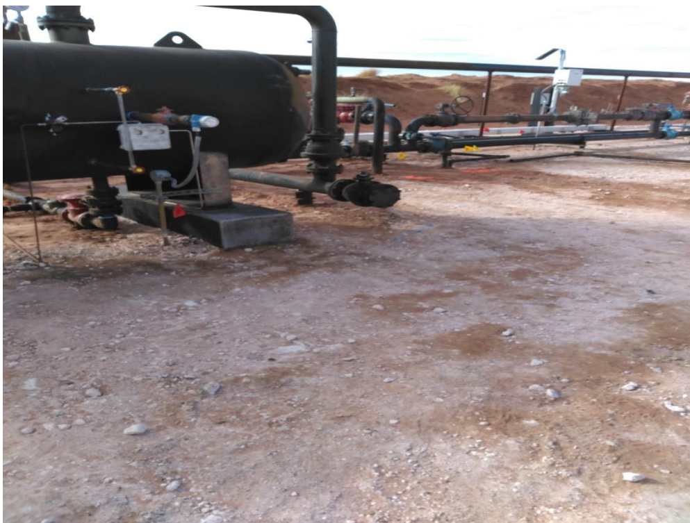
Photo 7: View of soil staining around vessels and ancillary equipment facing south-southwest
