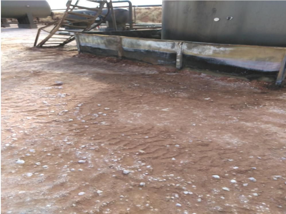
Photo 5: View of soil staining along the day tank's northern containment wall facing southeast
