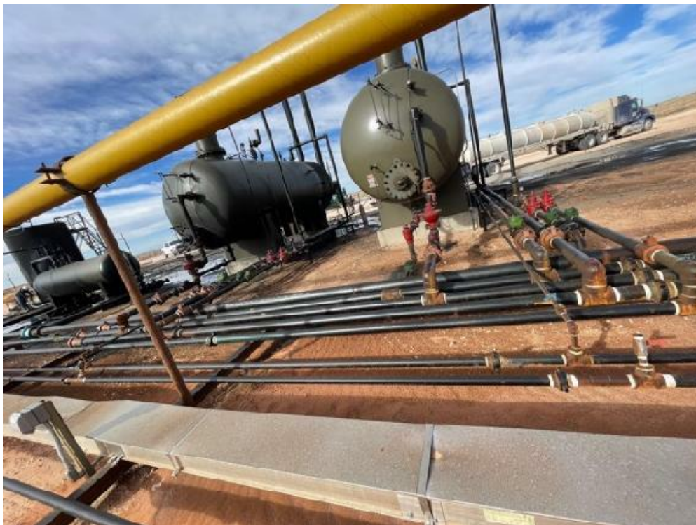
Photo 3: View of stained soil beneath piping facing north-northwest
