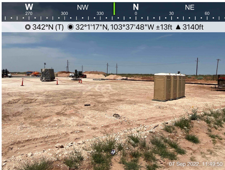
Impacted area viewing north/northwest, September 7, 2022
