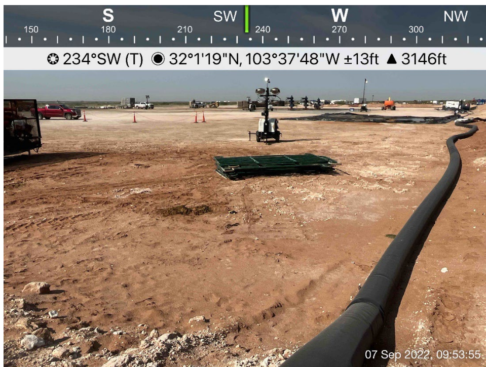
Impacted area viewing southwest, September 7, 2022
