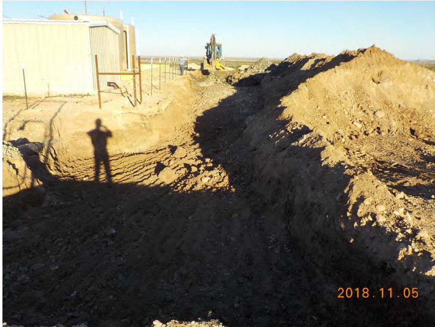
Photograph documenting initiation of site excavation activities in November 2018. View toward the east.
