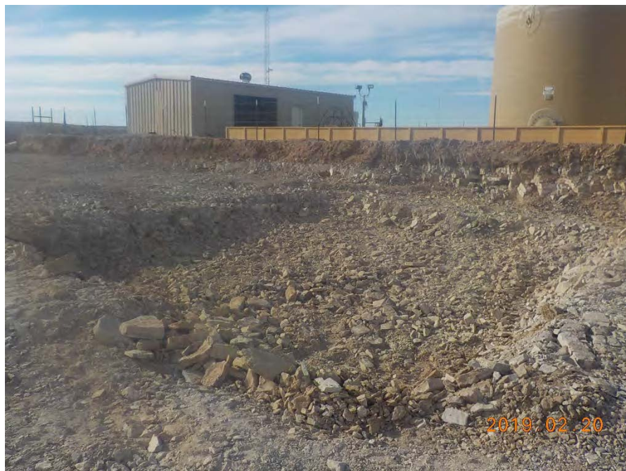
View of initial stages of excavation of the area with TPH RRAL exceedance (SS-10 area) that was ultimately excavated to approximately 6.5' in depth. View toward the northwest.
