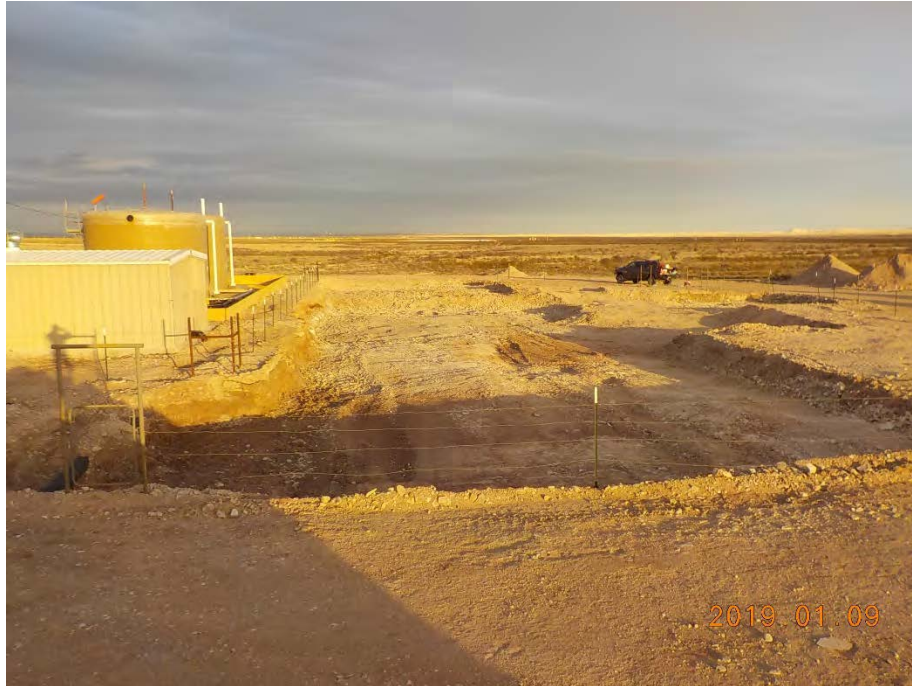
View of excavated area on January 9, 2019 prior to collection of soil cleanup confirmation samples. View toward the east.
