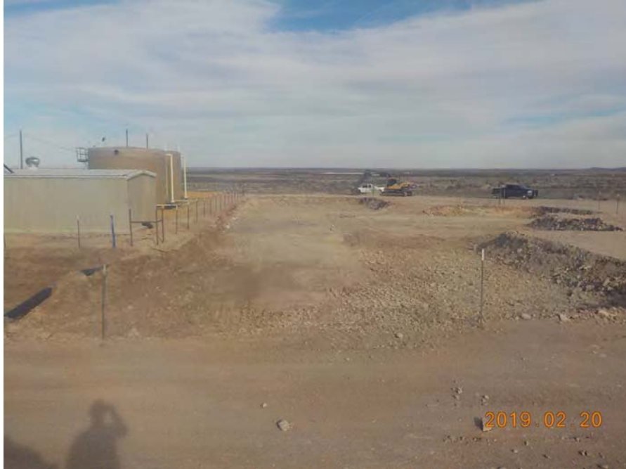
Photograph of final excavation prior to emplacement of liner and backfilling. View toward the east.
