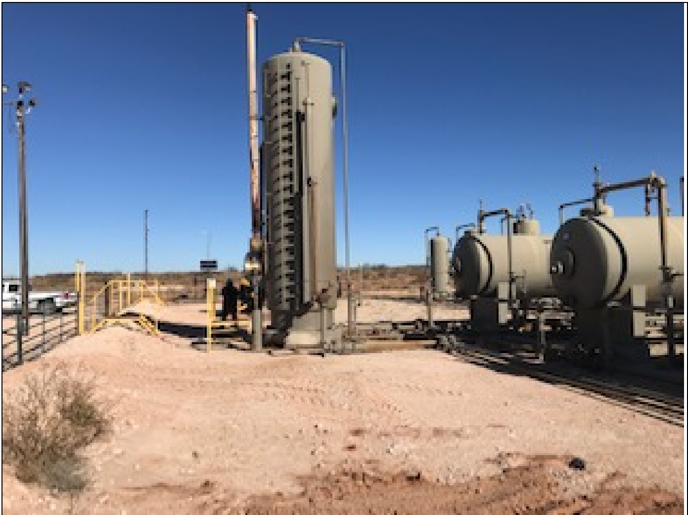
View north of heater treater area.
