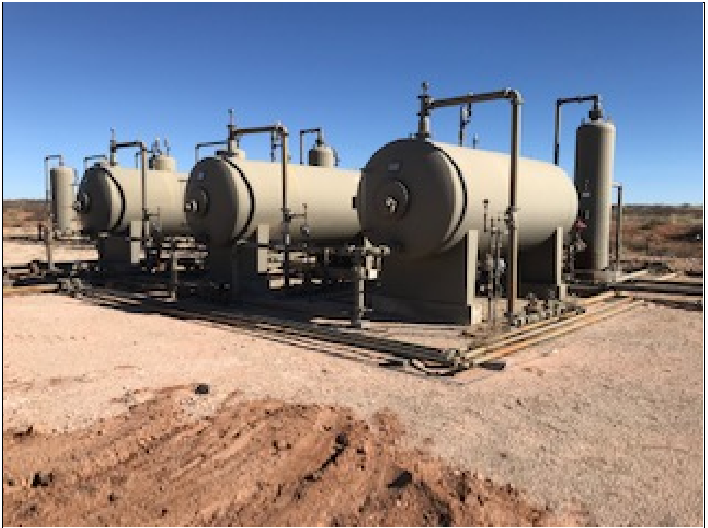
View east of process equipment.
