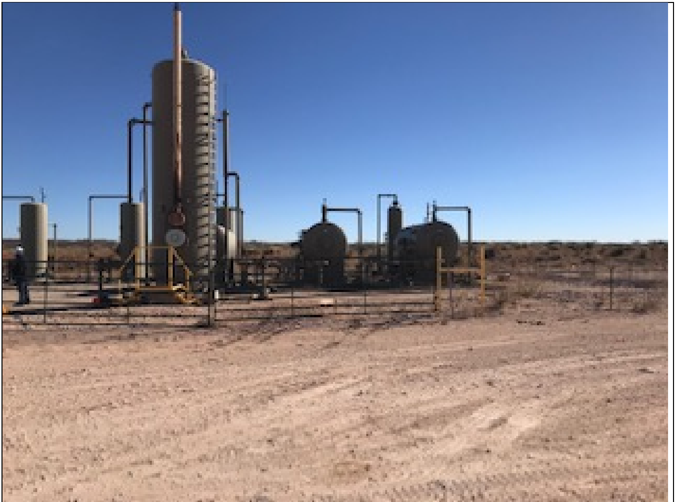
View east of heater treater area.
