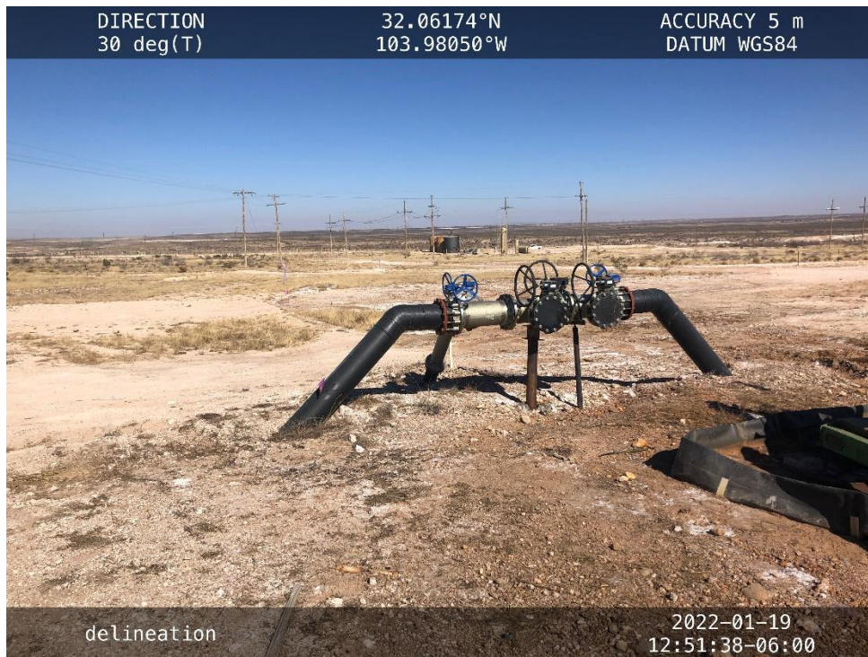
PHOTO 2: View of release from the top of the hillside.
