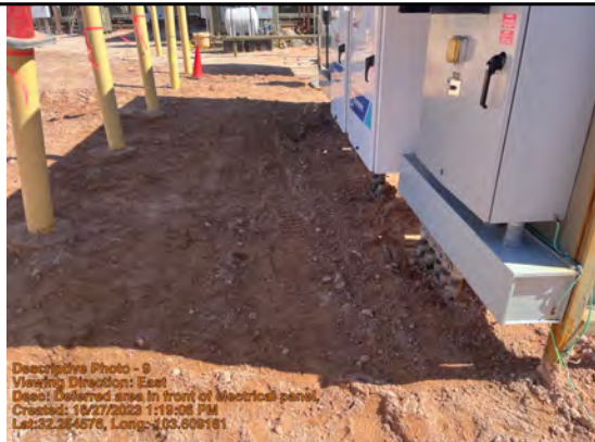
Deferred area in front of electrical panel.
