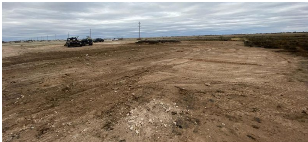
Figure 2: View of the release extent facing northwest from the southeastern extent of the release after surface scraping. Date Taken: 02/07/2023 12:31:15 GPS: 103.3704967°W 32.9140062°N
