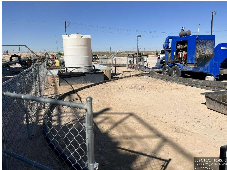
Area impacted by release on the pad, viewing to the northwest.
