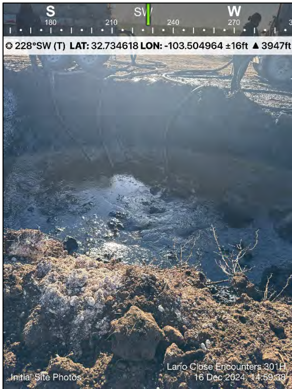
Photo 17: Initial site conditions, Iron House Draw
