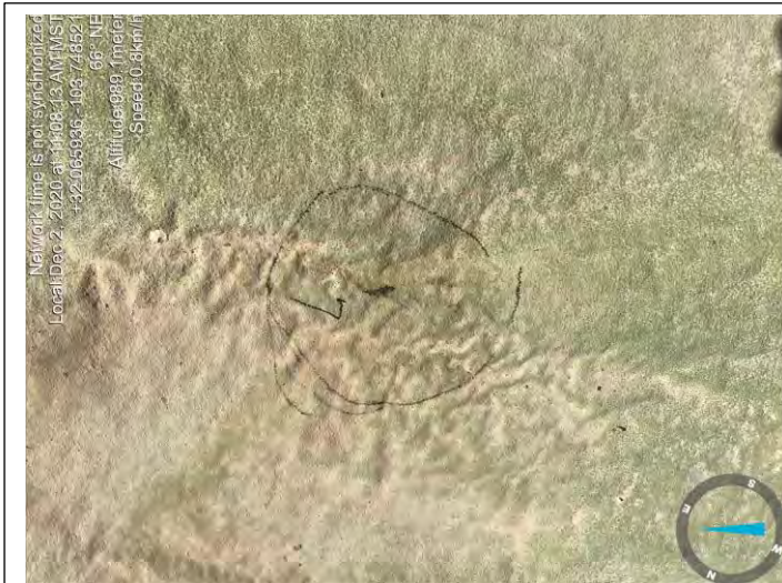
Hole in liner marked #7
