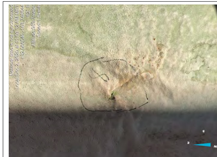
Hole in liner marked #8
