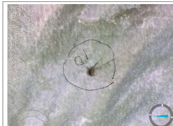
Hole in liner marked #10
