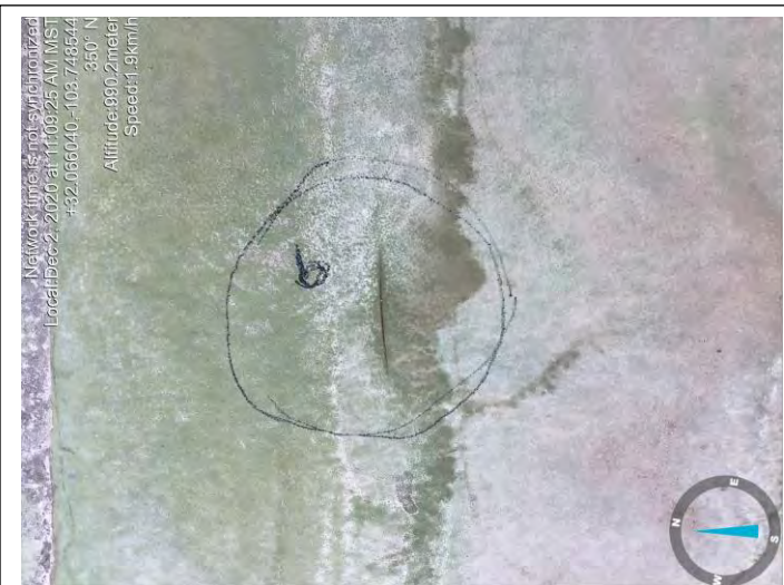
Hole in liner marked #9
