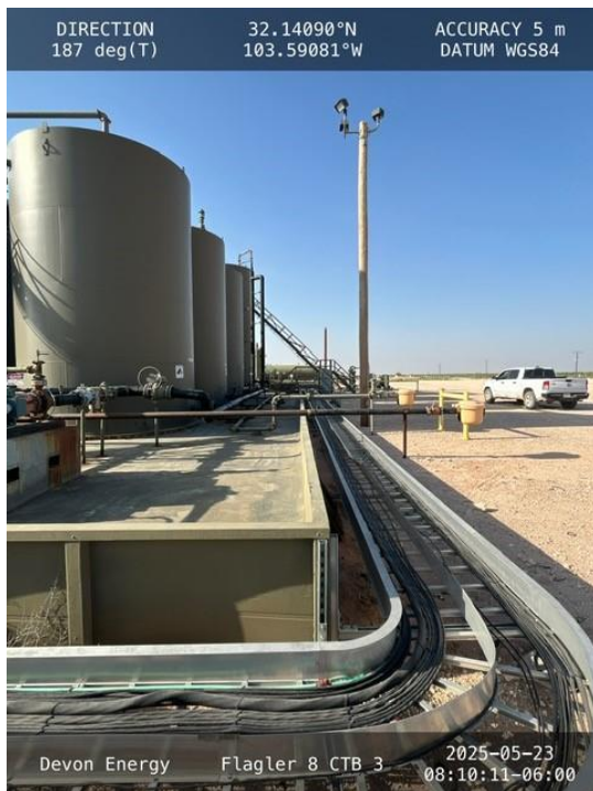
Photo 3 View of west side containment facing south.
