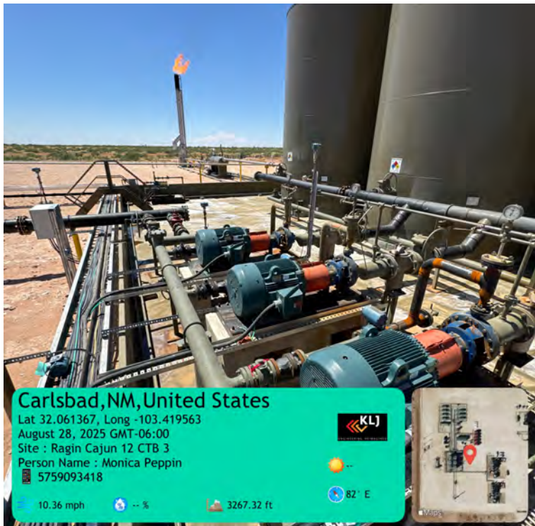
Southwest view of east area near water transfer pumps.
