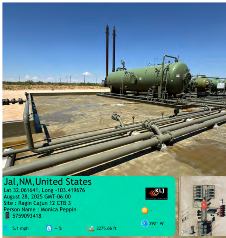
Middle area facing west near heater treater.
