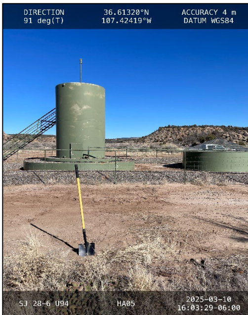
Photograph: 3 Date: 3/10/2025 Description: HA05 West of release, berm, and road View: East
