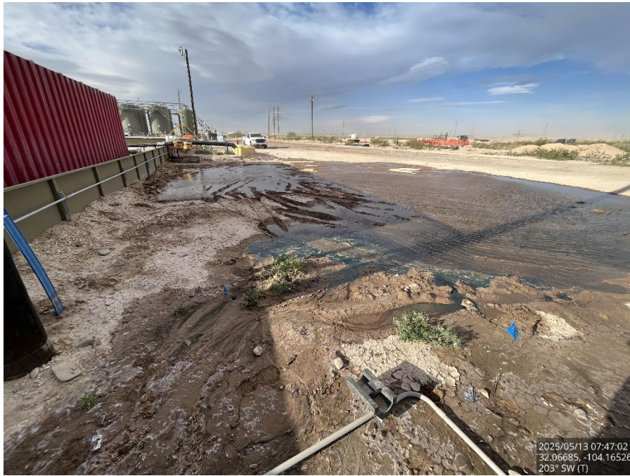
Spill area, viewing southwest.
