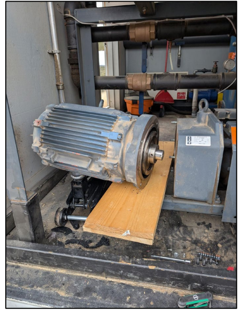
Photograph: 2 Description: Electric motor – removed from blower View: West
