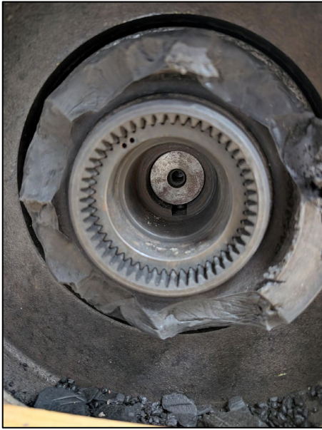
Photograph: 1 Description: Failed coupling, blower side View: NA
