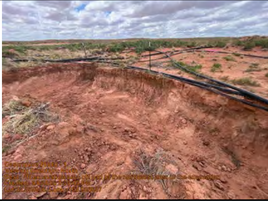
4ft excavation area off pad to the northwest area of the excavation. Field screened in compliance of criteria
