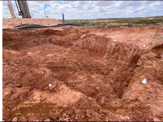
4.5ft excavation area excavated. The base field screens bellow criteria and the walls need further action
