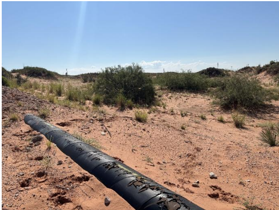
Figure 18. Exposed oil pipeline within dune blowout
