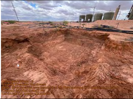
6ft excavation area benced at 4ft. Field screens in compliance of criteria
