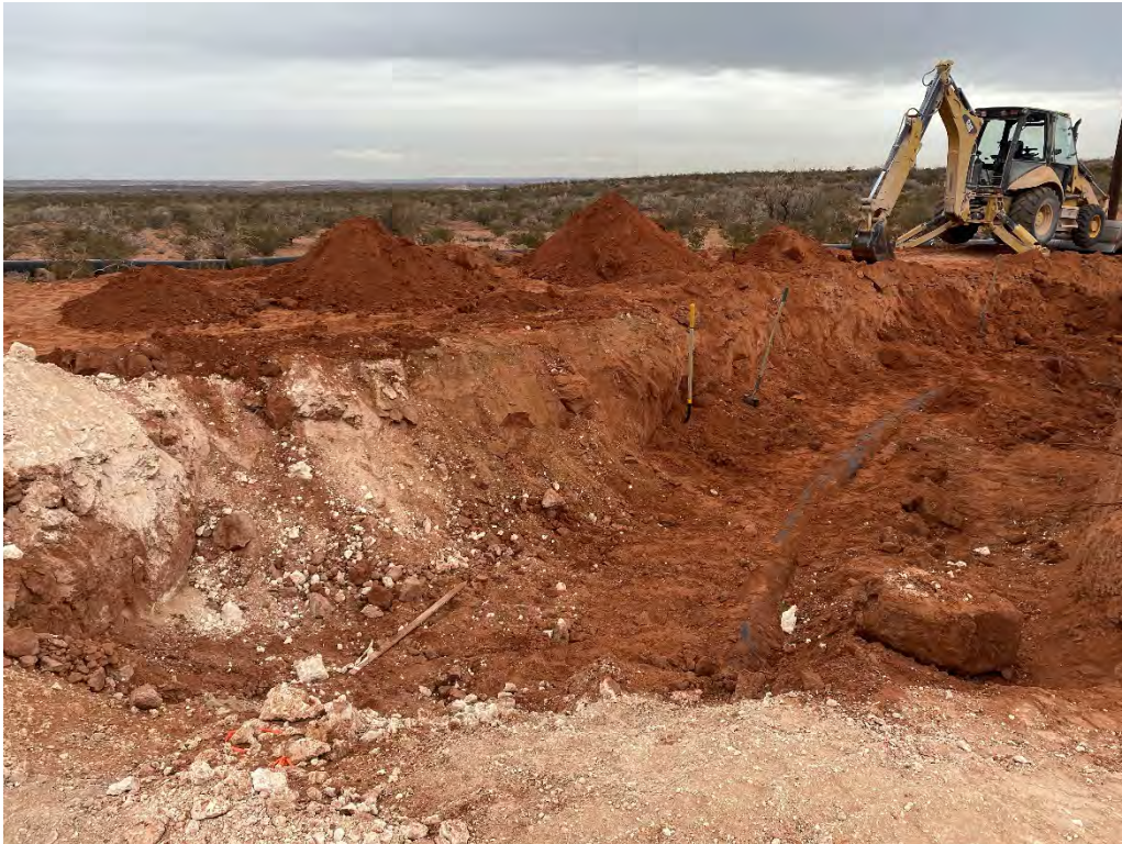
Photograph 3: View northwest of excavation along the lease road. The excavation was disruptive of nearby operations.
