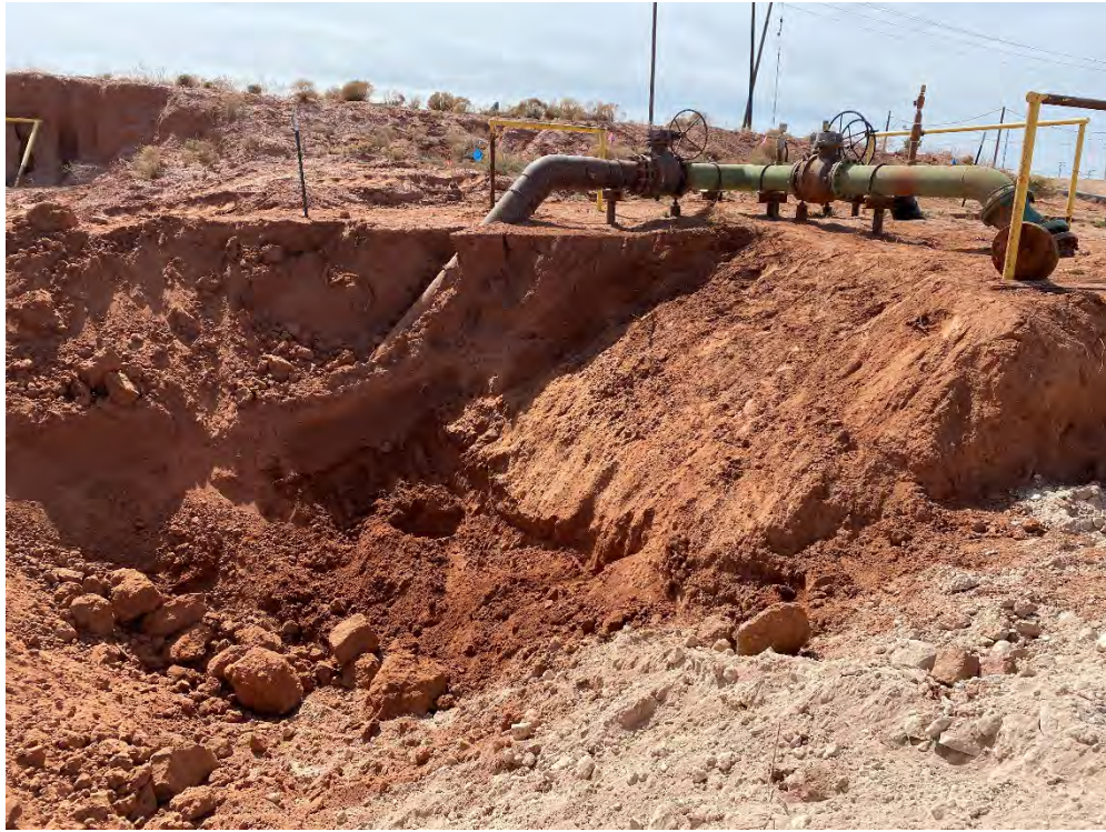
Photograph 1: View southeast of the above ground production equipment adjacent to sidewall SW08.
