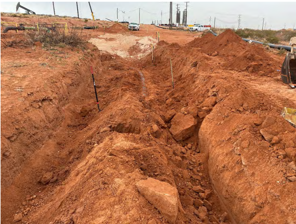
Photograph 4: View south of excavation along the lease road. Note the SWD riser equipment and the frac operation visible on the adjacent pad in the background.
