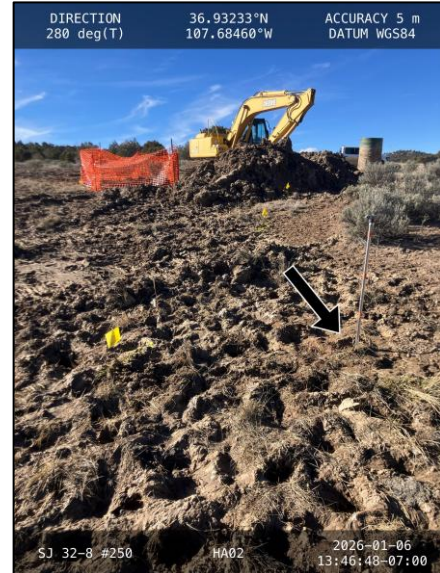
Photograph: 2 Date: 01/06/2026 Description: Hand auger boring, HA02, advanced within the release footprint. View: West
