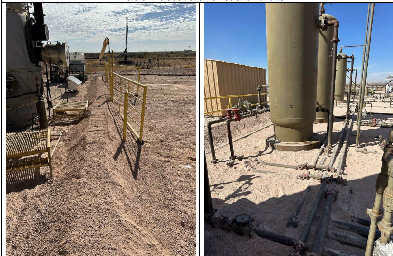
Photos of the site following the completion of the remediation and backfill
