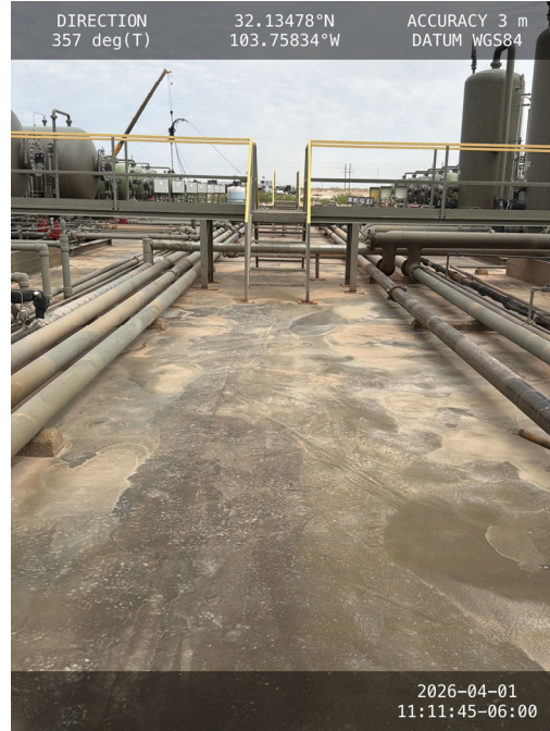
Photo 10 Photo of containment towards north.
