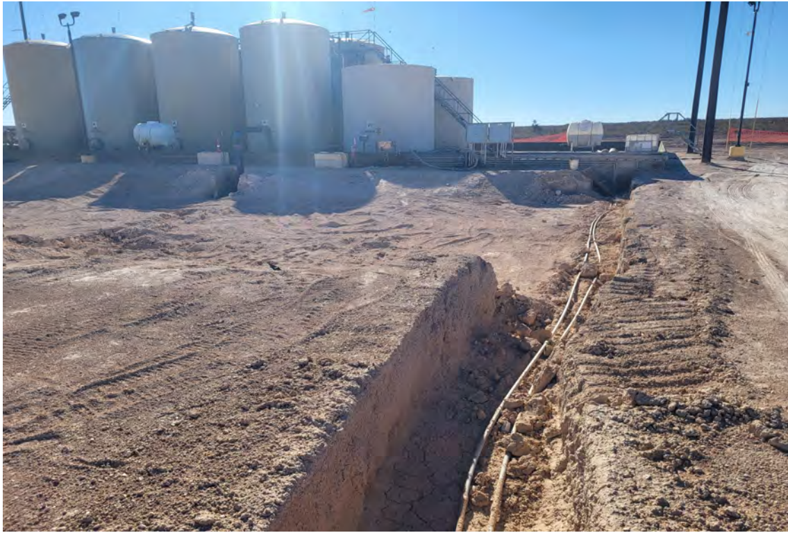
Pipe and electrical trench 25' long 4' wide and 3' deep against the battery 90' long 35' wide and 2' to 2.5' deep
