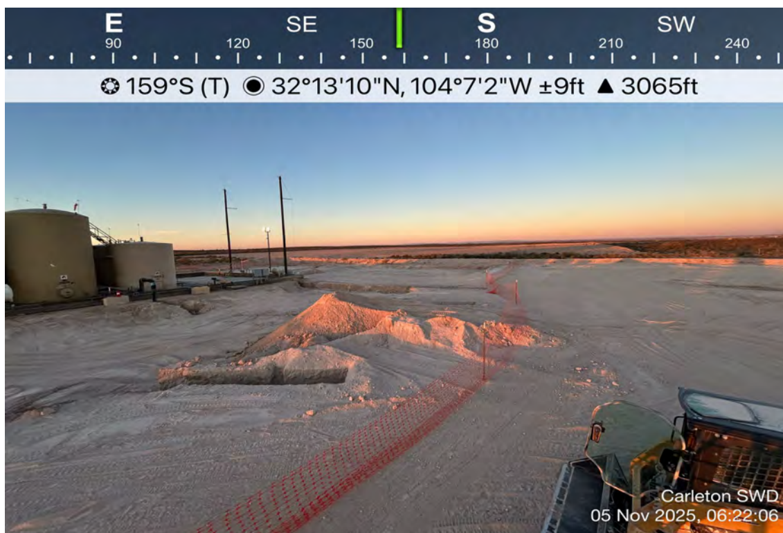
East side of excavation trench is 3' deep and approximately 5' wide approximately 1.5' to 2' deep and 70' long, and 30' wide
