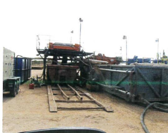
Above: Centrifugal Closed Loop System
