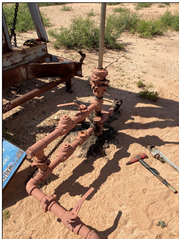
3) Twin Lakes SA #099 (30-005-61261) – Wellhead
