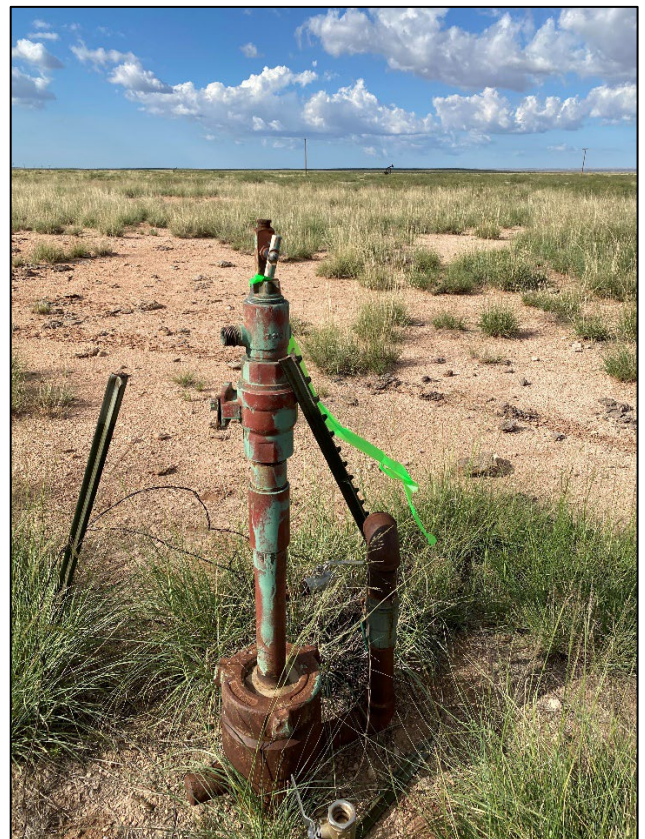
4) DLQ #04G (30-005-60080) – Methane Monitoring Complete
