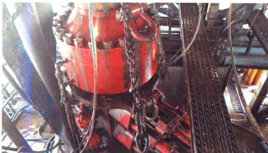
Figure 1: Winch System attached to BOP Stack
