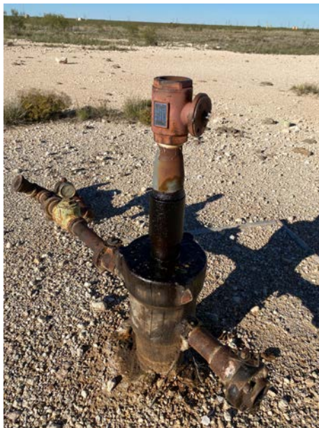
Shelly State #006 Leaking Wellhead
