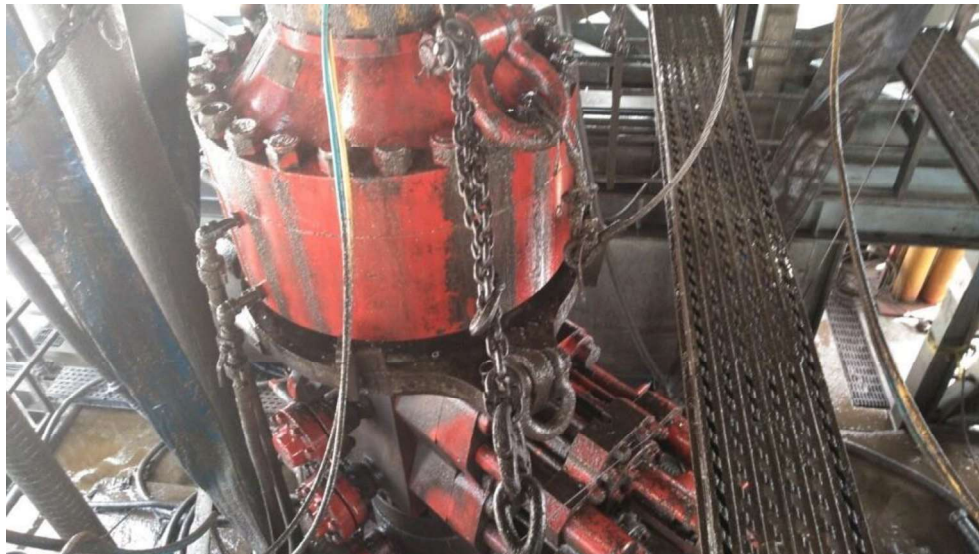
Figure 1: Winch System attached to BOP Stack
