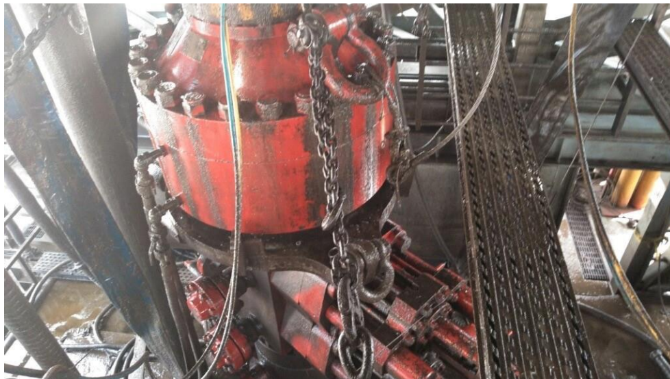
Figure 1: Winch System attached to BOP Stack
