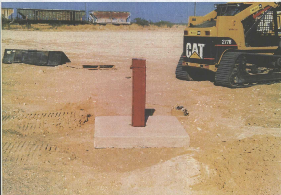
MW-8A above ground vault.
