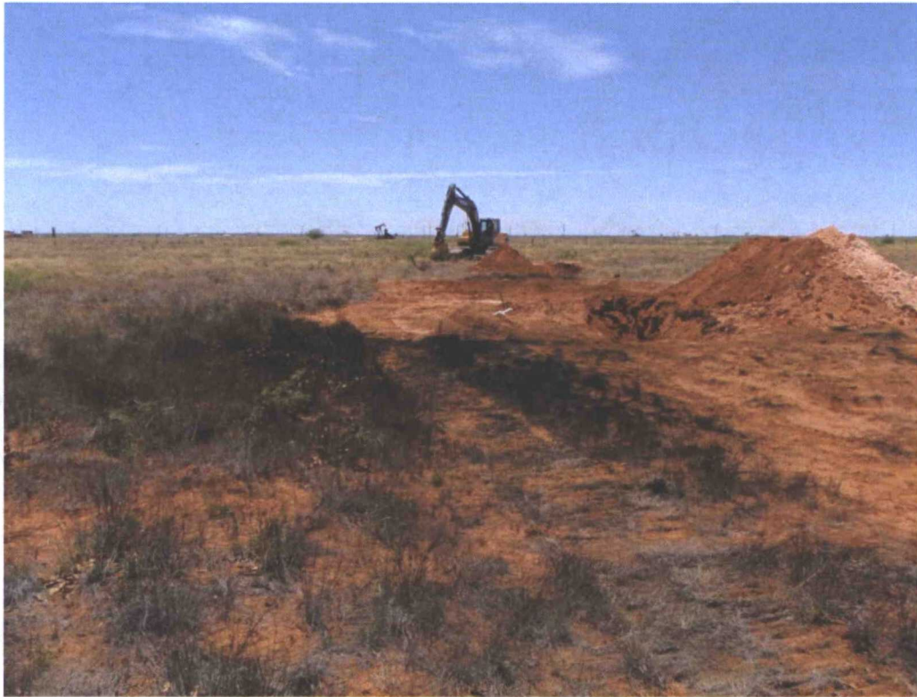
Surface staining from initial release at the Line 4A Release Site. (Looking North)
