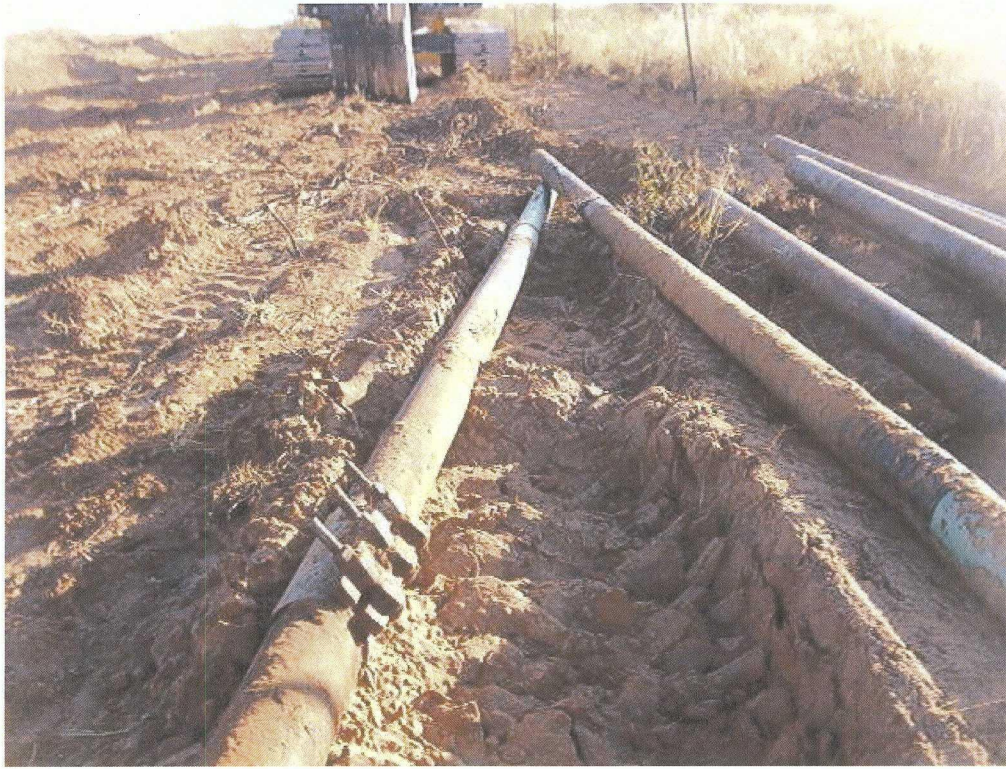
Photograph 5: Clamp on pipeline and relatively new section of green pipe.
