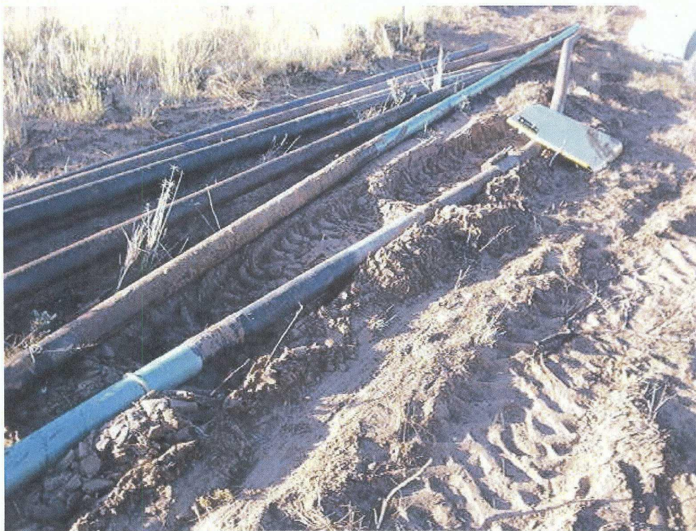
Photograph 6: Clamp on pipeline and relatively new section of green pipe.
