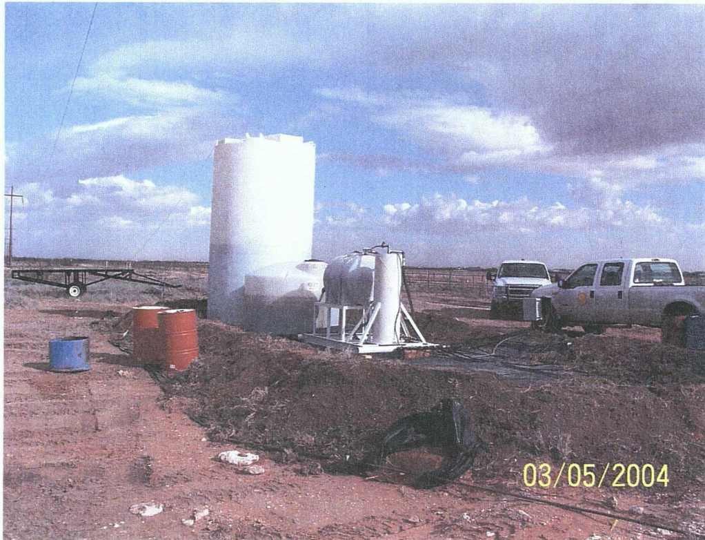
Photograph #5- Looking easterly at recovery system.
