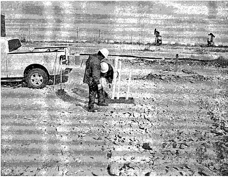
Figure 3: Bentonite being placed around Lysimeter 1 casing and associated Tensiometer casings. MW-1 is visible to the upper right of Lysimeter 1 casings.
