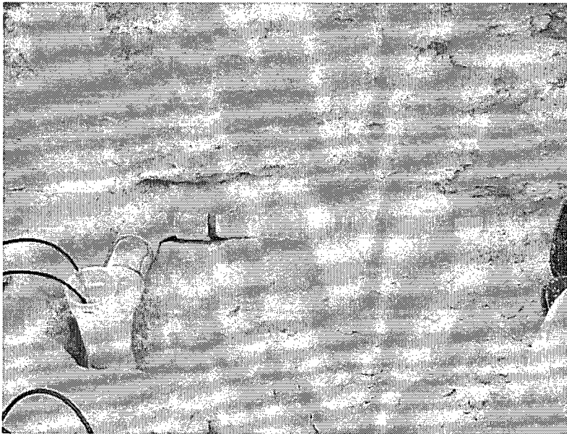
Figure 1: Lysimeter 2 with fill material during installation. Slotted collection pan is in trench dug under intact vadose zone material.
