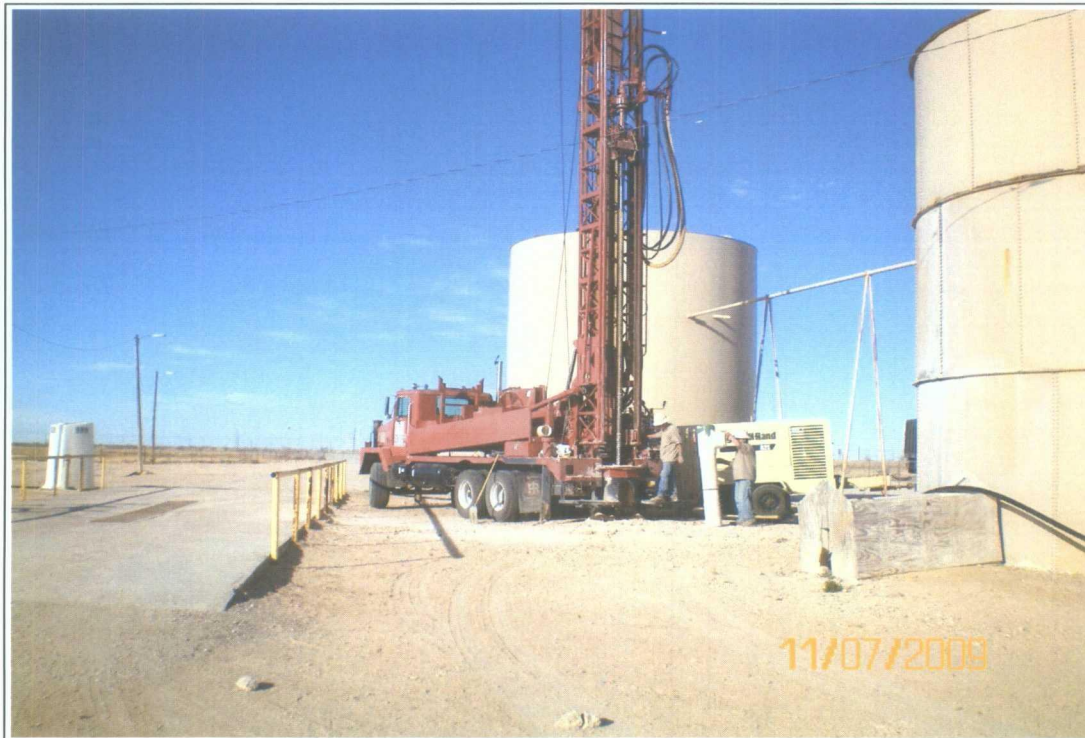
1. Location of recovery well RW-1 at the brine pond area (view to the north).
