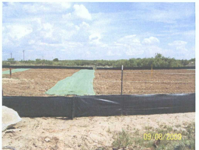
Completed site restoration with silt netting and Excelsior Green to hold seed in place 9-8-2009
