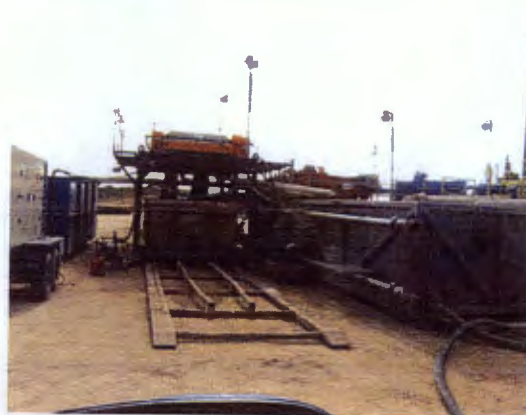
Above: Centrifugal Closed Loop System
