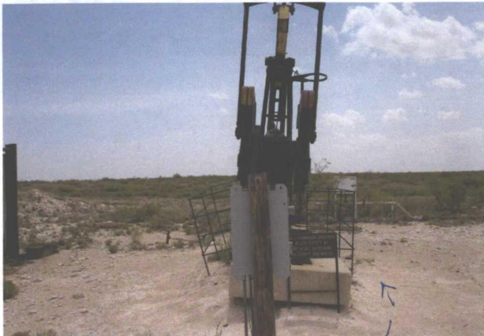
PUMPING UNIT LEANING →
