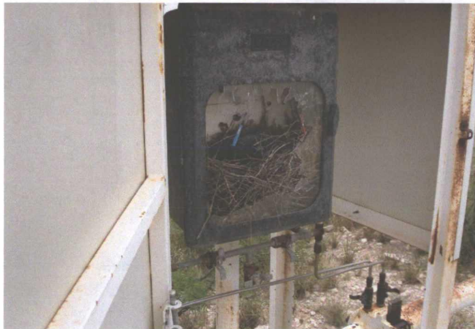
METER ON LOC. NON-OPERATING.
