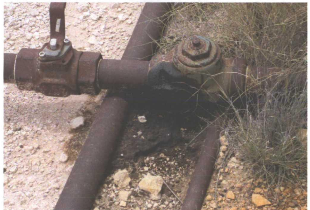
CHECK VALVE LEAKING
