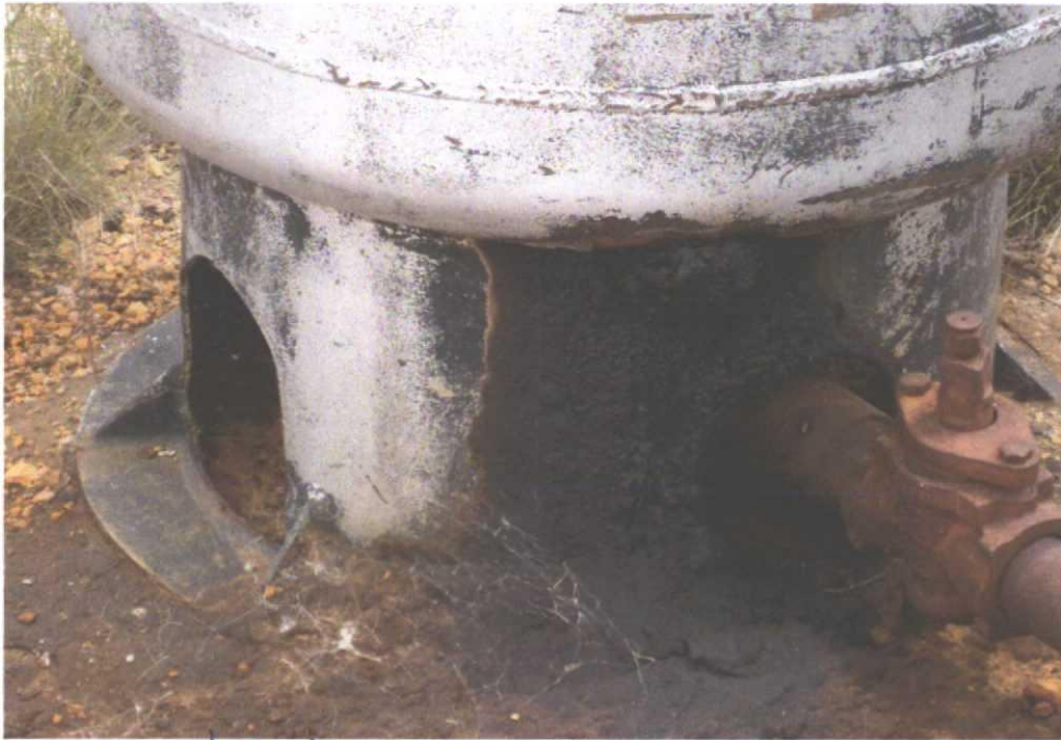
VESSEL ON LOC LEAKING ↑
