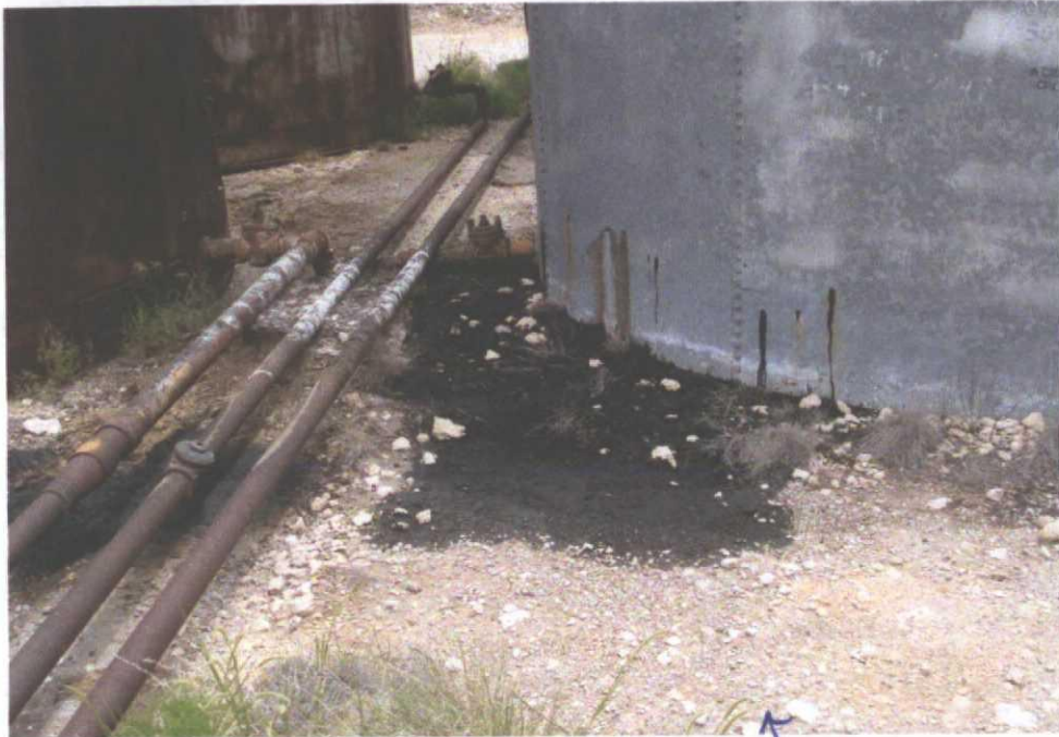
SW TANK LEAKING ↘
