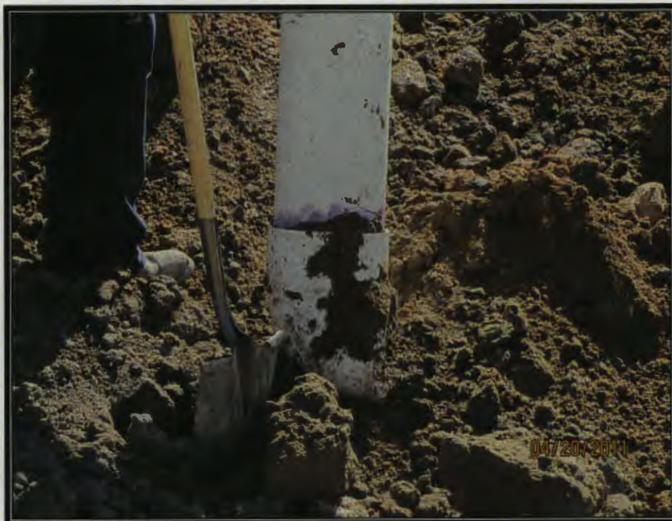
Photo 5: Bottom of Leak Detection System, No Concrete Found
