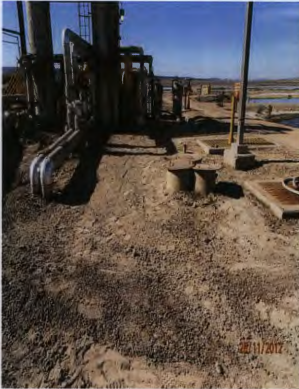
East side of the benzene strippers
