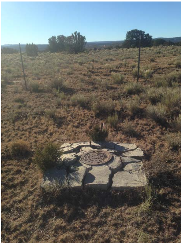
Photo 3. Photo facing south, toward MW-5-24B of well pad broken up for removal.
