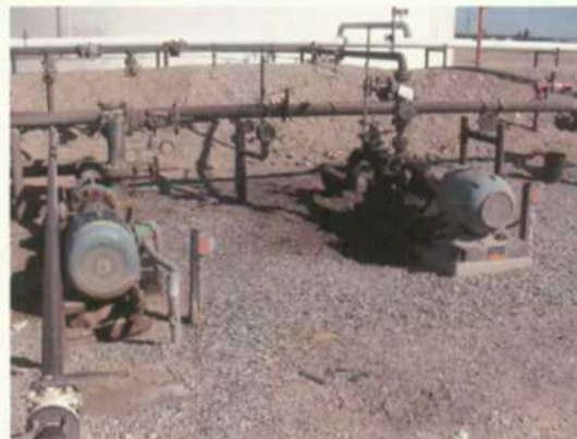
Pic #6- 437 Crude oil tank transfer pumps. Needs containment.
