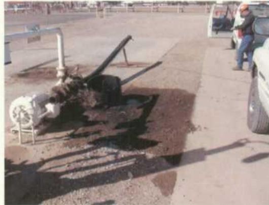
Pic #5- Crude oil Lact unloading area needs containment.
