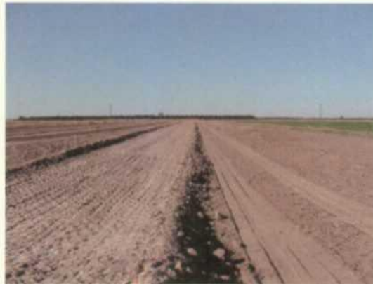
Pic #9- SE corner of south plant farm area. Picture looking north. Area being prepared for new stormwater berm.
