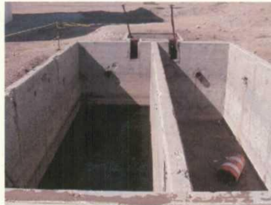
Pic #10- Old API separator located near the south side asphalt tank farm. Requires closure. Standing fluids.
