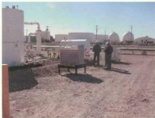
Pic #3 - Pipeline pump area. Chemical tote tanks need containment.
