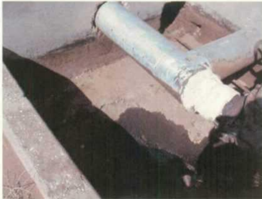
Pic #8- Gas-Oil transfer pumps sump. Bottom of sump has lost integrity.
