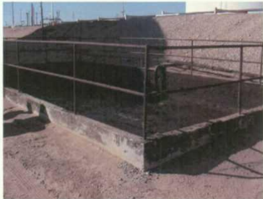
Pic #2- Tank 437 water draw sump. Out of service. Requires closure.
