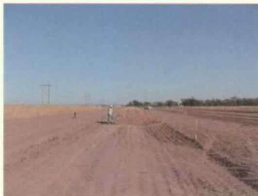
Pic # 10- North side of south plant farm area. Picture looking east at new stormwater berm being built.
