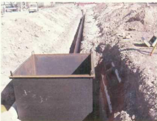
Pic #18- Same as above. Navajo needs to submit design information for OCD approval and include in Discharge Plan.
