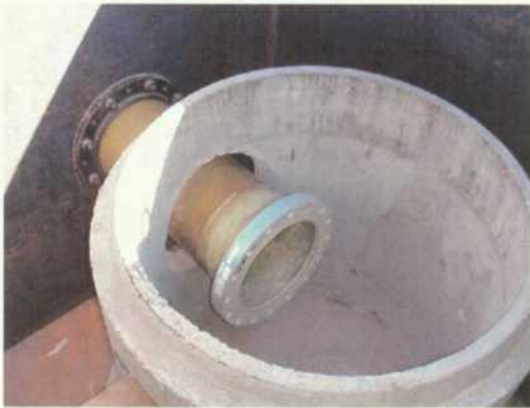
Pic #17- New wastewater system for new north side Gas-Oil Hydro-treater.
