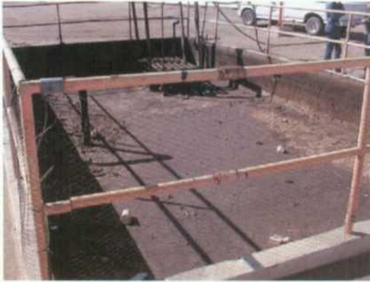
Pic #7- 439 water draw sump. Out of service. Requires closures.
