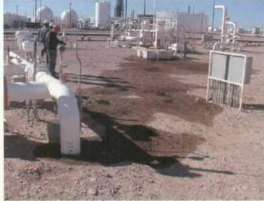
Pic #4- Crude oil pipeline pump area spill. Sump overflowed oil.- Requires action.
