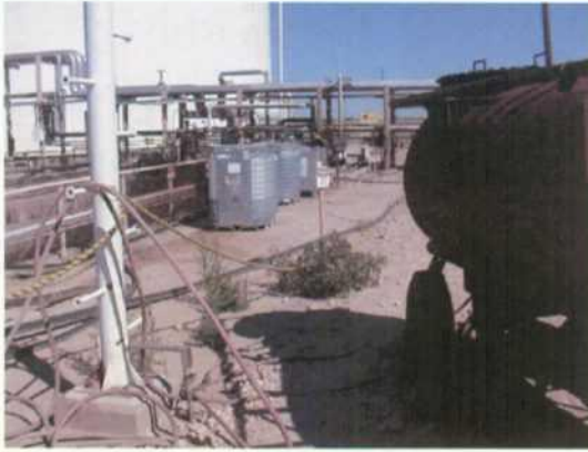
Pic # 16- AST's chemical tote tanks located next to Main API Separator needs containment.
