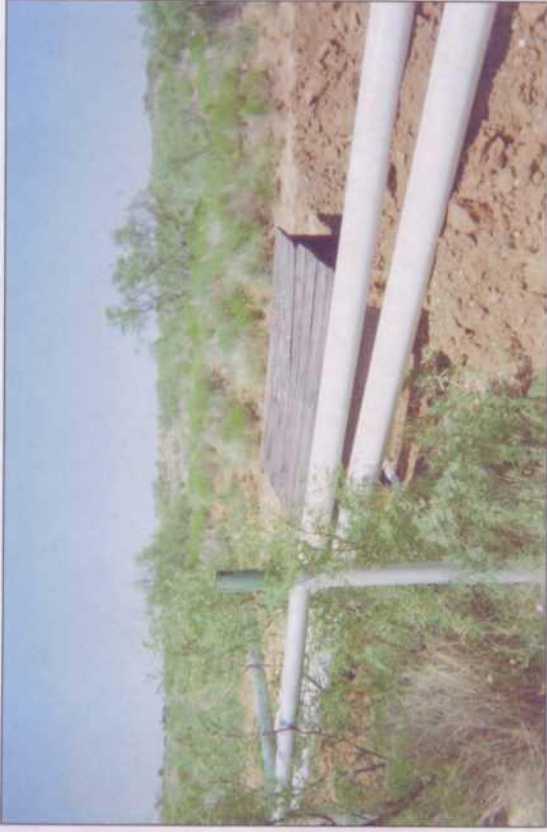
undisturbed junction box
