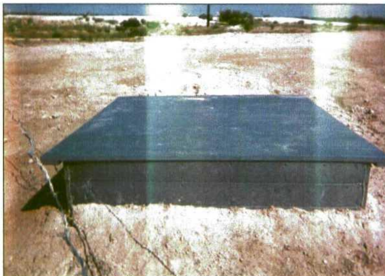
New Junction Box
